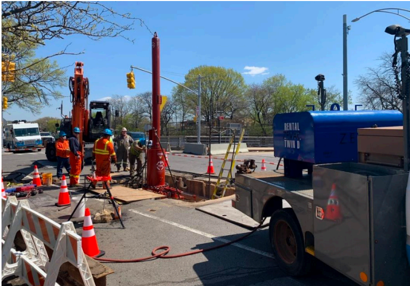
Figure 7: ZEVAC in use during a pipeline repair involving old pipe that has significant water and oily sludge inside the line.
