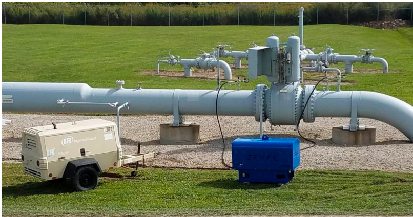
Figure 6: ZEVAC in use at a pigging receiver that is susceptible to receiving high levels of liquid and solid debris.
