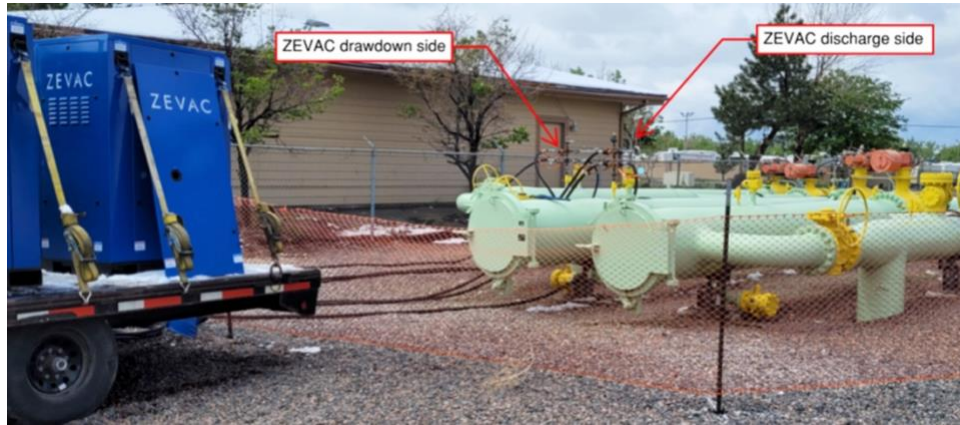
Figure 35: ZEVAC equipment setup
