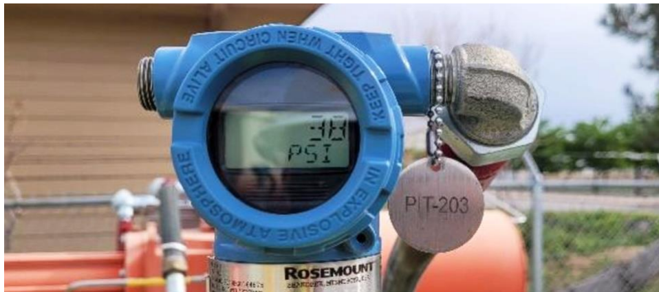
Figure 34: Pressure indicator after drawdown
