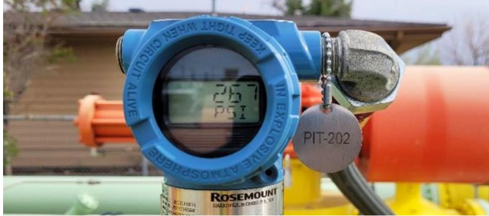
Figure 33: Pressure indicator before drawdown
